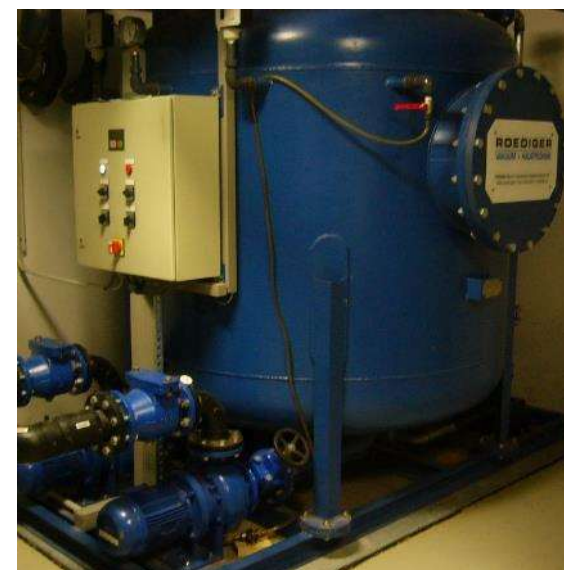
Vacuum Pumping Station for Blackwater
