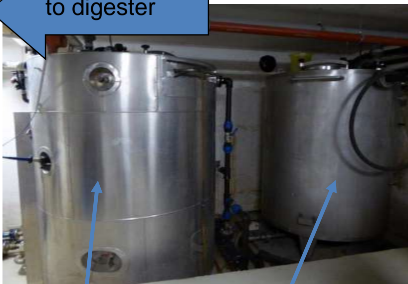
Sanitation/Higienisation and Mixing of Biowaste and Blackwater
